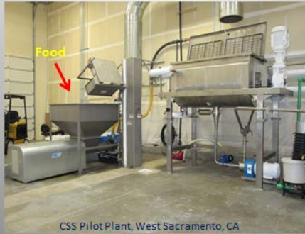
CSS Pilot Plant, West Sacramento, CA
